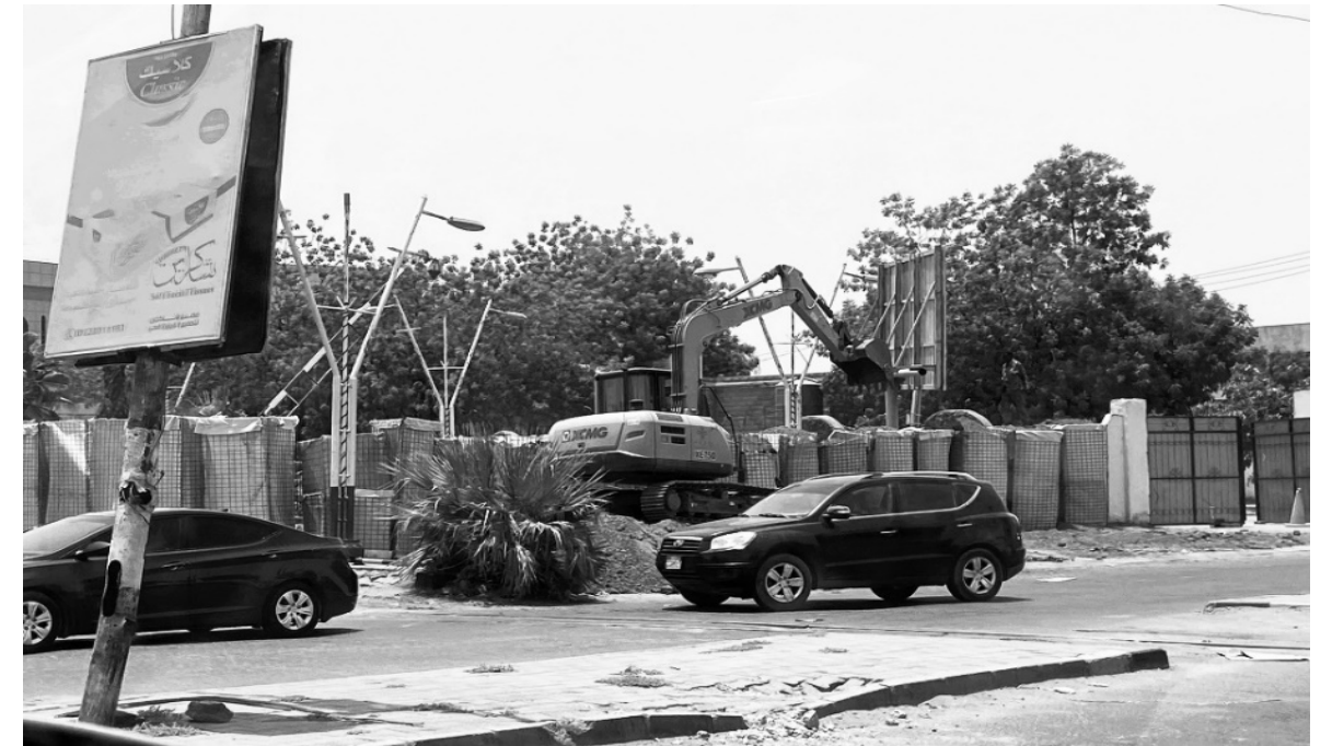
Figure 1: crane filling fortification by sand to surround the military headquarter in Khartoum in early June 2021
